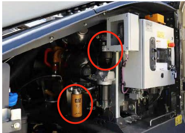
Important service points located on the ground level and easily accessible .
