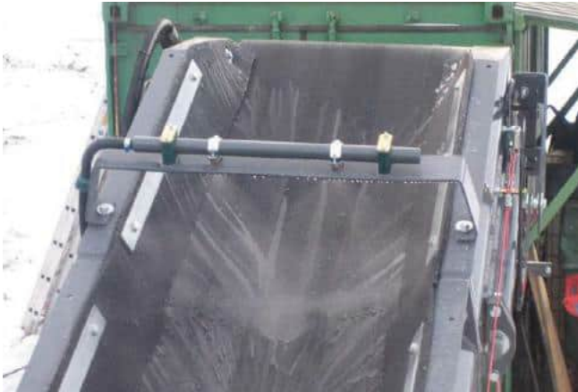
High pressure water spraying system for binding dust particles. Nozzles located on main conveyor and crusher's feed hopper.
